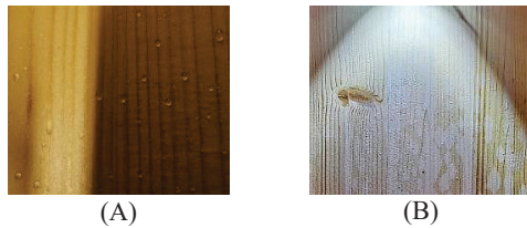
Figure 9. Water droplets occurred on the CLT-element treated with the FR-stain during the absorption step (A). The discoloration of the surface (B) appeared in the beginning of the absorption step but quickly disappeared again.
