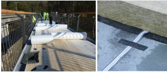
Figure 9: Bridge Ruppertsweil, application of sensor band on the wooden panel of a timber bridge (left) and detail of sensor band (right)
