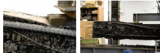
Photo 3: Partial compressive deformation around loading plat
