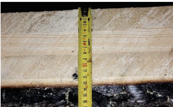
Figure 19: Charring in the middle of the CLT span.
