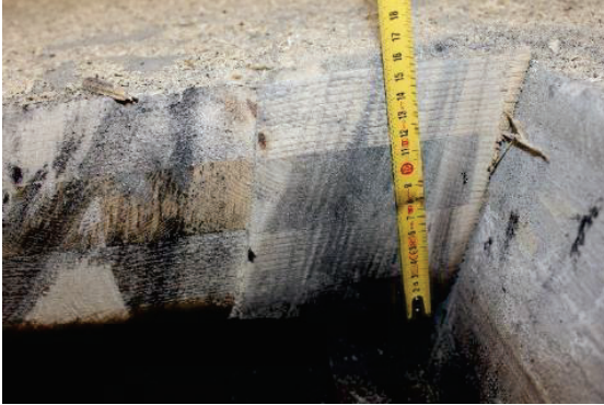
Figure 18: Charring in the DELTABEAM® and CLT slab joint, next to the joint concrete.
