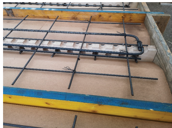
Figure 10: Specimen with the steel mesh and the rebars positioned in the area of negative bending moments.
