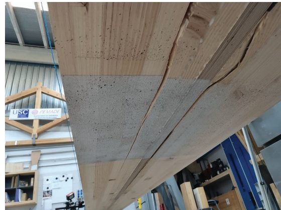
Figure 9: Longitudinal failure of the glulam flange
