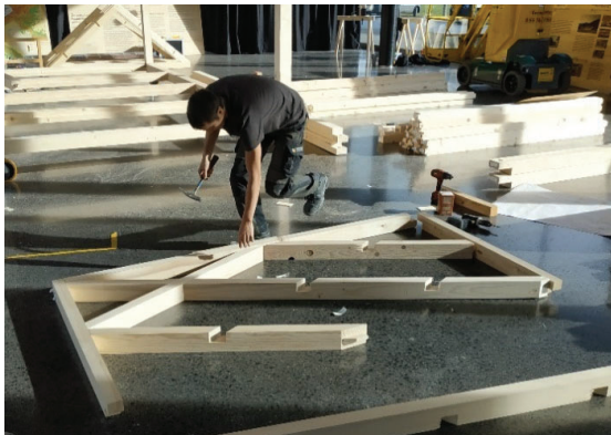
Figure 2: A carpenter assembling the wooden frame. The complicated connections in the frame are still visible.
