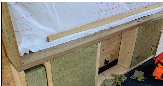
Figure 6: Sensor under window. © Kruse Smith
