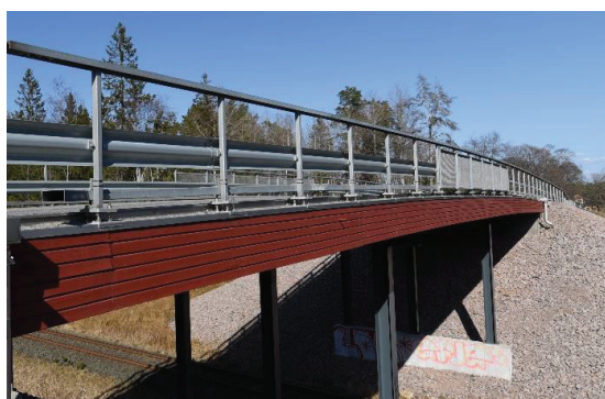
Figure 25: A typical stress-laminated timber bridge over railroad. Built 2017 in Hörle, Sweden, by Moelven Töreboda. Photo: Per-Anders Fjellström.
