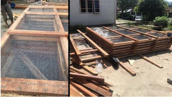
Figure 6: Prefabrication of timber and chicken wire wall frame modules at the workshop in Palu.
