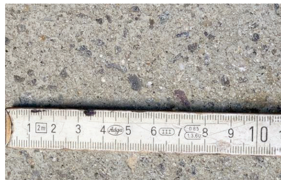
Figure 5: Sandblasted underside of the prefab concrete part
