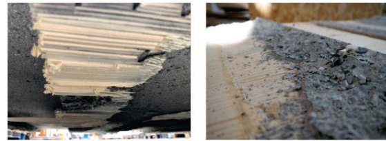
Figure 9: Bond failure in the timber and the concrete substrate, as predicted from the calculation.
