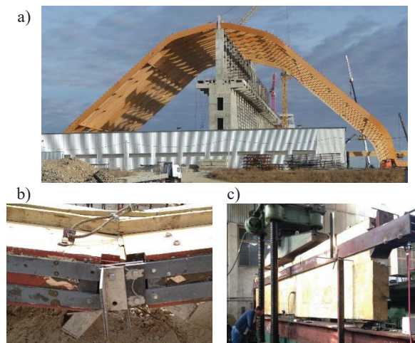
Figure 7: 87.2 m span warehouse arches: a - frame assembly; b - joint of collapsed arch; c - joint testing
