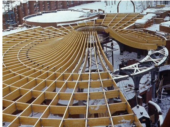
Figure 3: Radially arranged multi-span beams of the Lipki boarding house roof with rigid joints on inclined glued-in bars (1985): a - structural scheme of the girder; b - installation of roof beams
