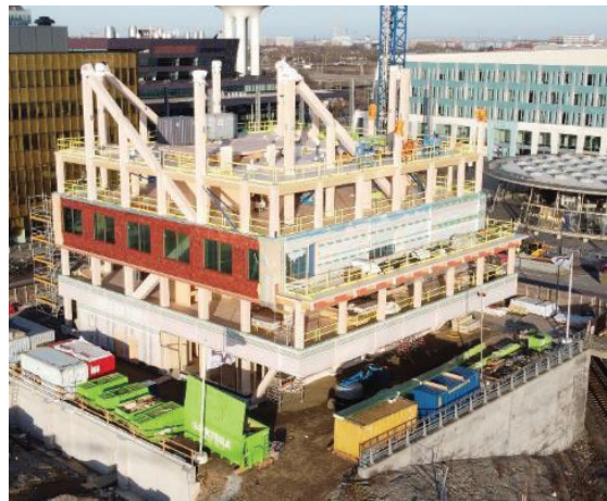
Figure 16: On site situation the 21 st of February. Picture taken from south-west. Timber structure levels 1 to 4 is completed.
