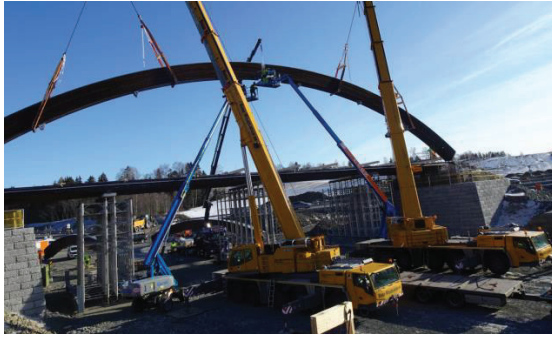
Figure 13: The glulam arches are assembled on the construction site. Picture taken by Sweco
