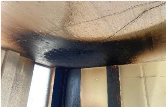
Figure 13: limited damage to the ceiling structure
