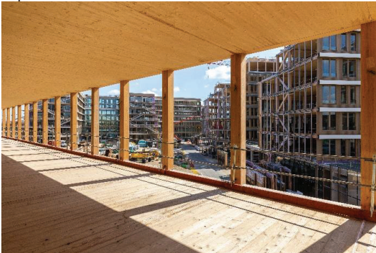
Figure 2: Erection of CLT slabs meant to remain visible in the project © Raffin
