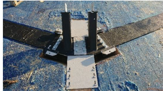
Figure 17: Detail of the base of the compression strut on the tension ring – tension ring and steel connector
