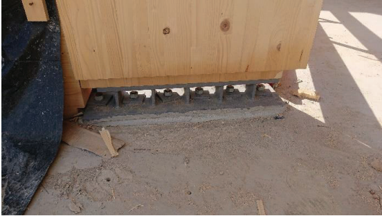
Figure 19: Detail of the base of the foyer column with special steel part and glued-in threaded rods
