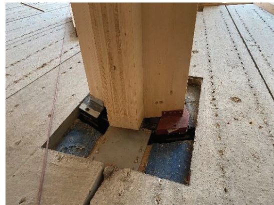
Figure 18: Detail of the base of the compression strut on the tension ring – including wooden column
