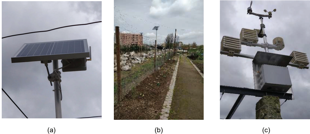
Figure. 2. Data acquisition subsystem: (a) detail of peripheral tower with the solar panel to feed the battery and the antenna; (b) peripheral tower installed in the urban garden near the river flow; (c) main tower with the meteorological station.
