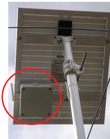
Figure. 7. Omnidirectional antenna installed in the peripheral towers.
